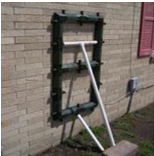
Fig. 39. Cutting an opening in the wall by means of the detonation straps [30].
