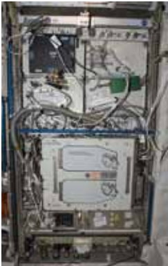
Sub-rack-sized experiments with standard utilities such as power, data, cooling, and gases.
